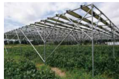
Exterior of the power generator
