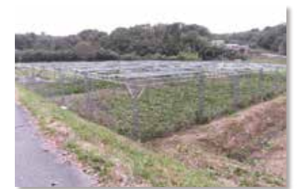
Exterior of the power generator
