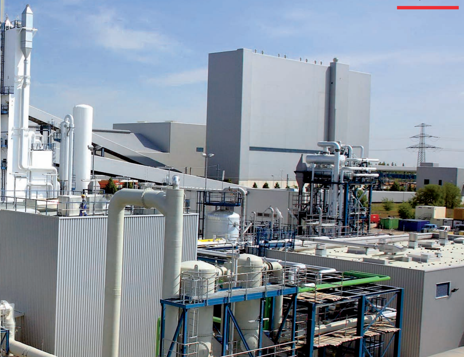
Carbon capture and storage technology: boiler assembly for pilot plant at Schwarze Pumpe, Germany
