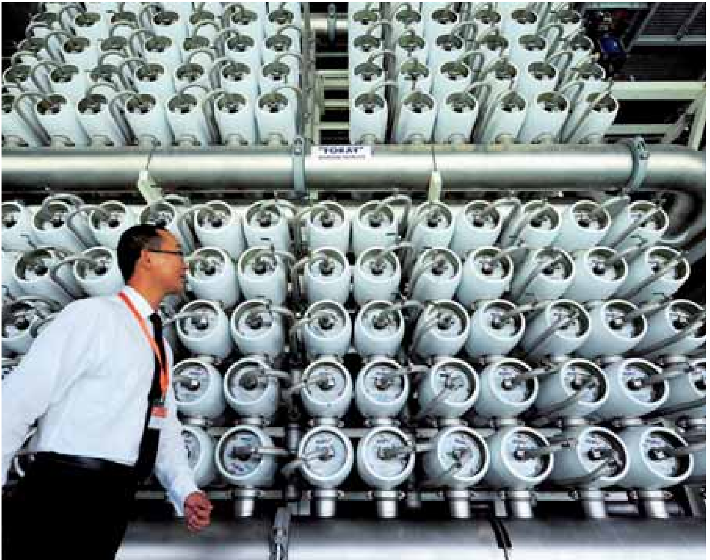
An engineer inspects membranes used in the treatment of recycled water, in the newly opened Sembcorp NEWater plant in Singapore
