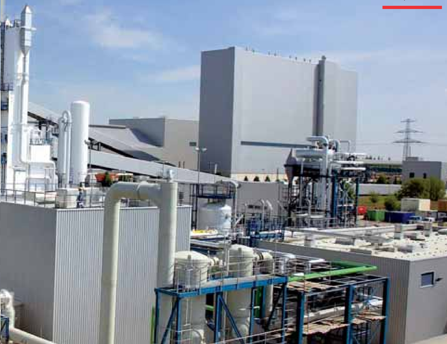
Carbon capture and storage technology: boiler assembly for pilot plant at Schwarze Pumpe, Germany
